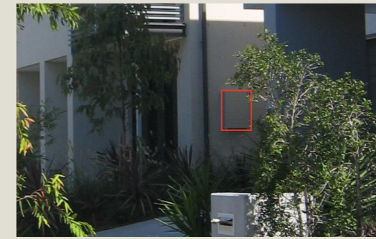
2.9 Electrical Meter Box on side building wall
